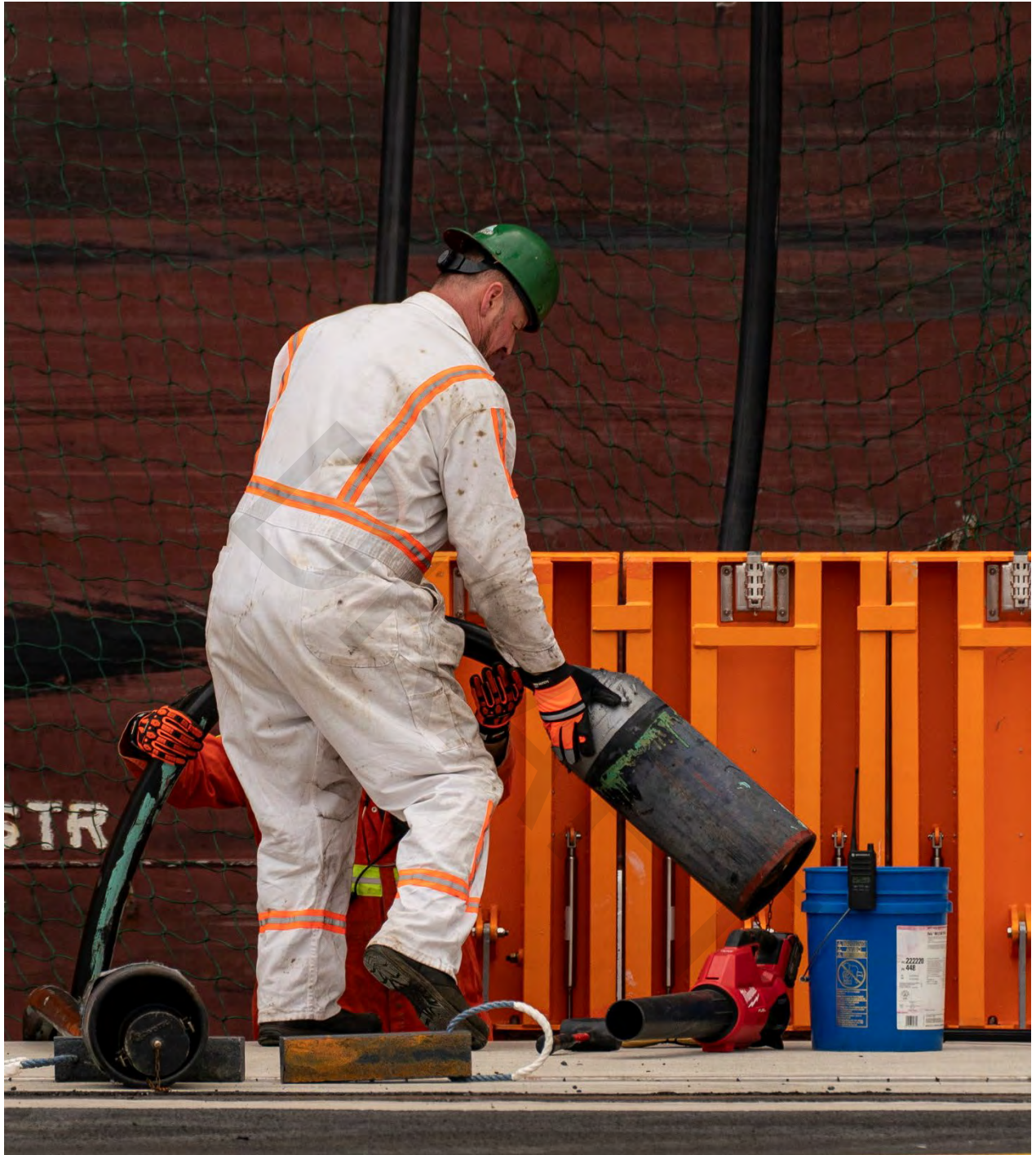
Longshore worker connecting an MSC vessel to shorepower at Terminal 5 in the North Harbor.
